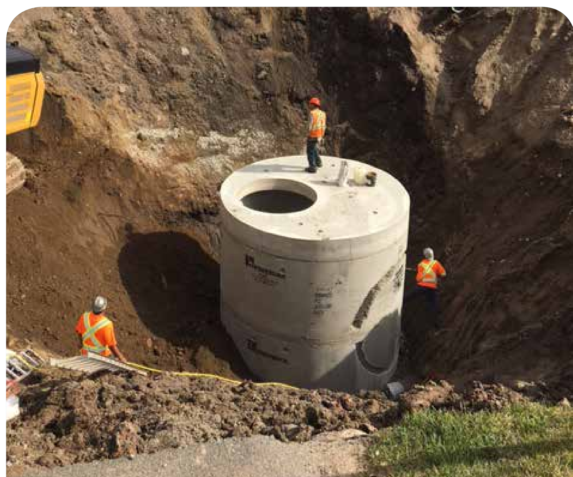
Storm sewers - 283 km
